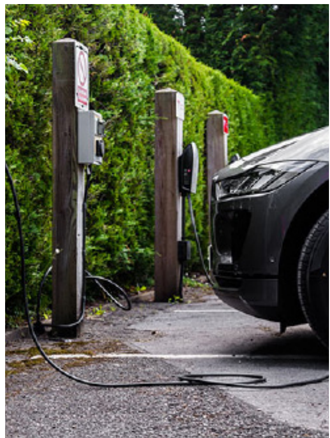
Figure 136: EV Parking should not be intrusive and should not detract from the character of the area.
