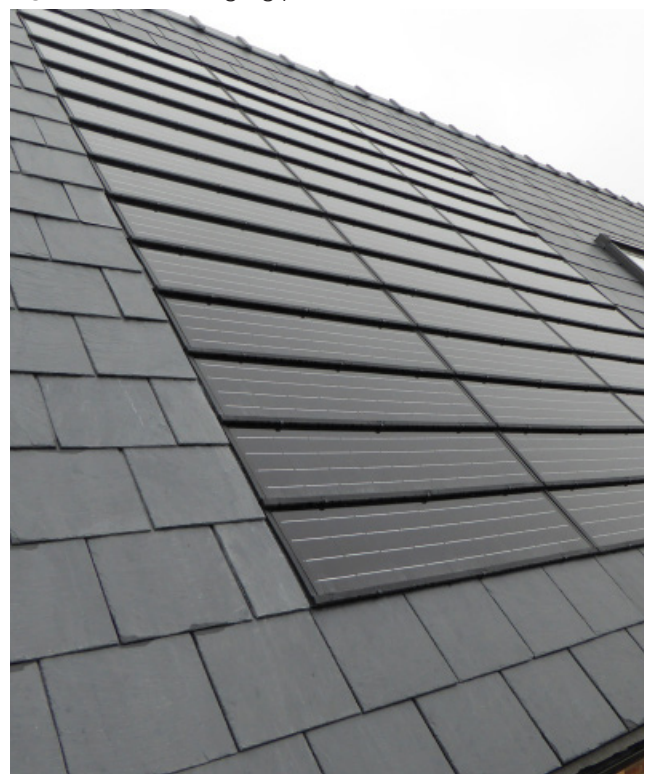
Figure 120: Integrated PV panels on roof
