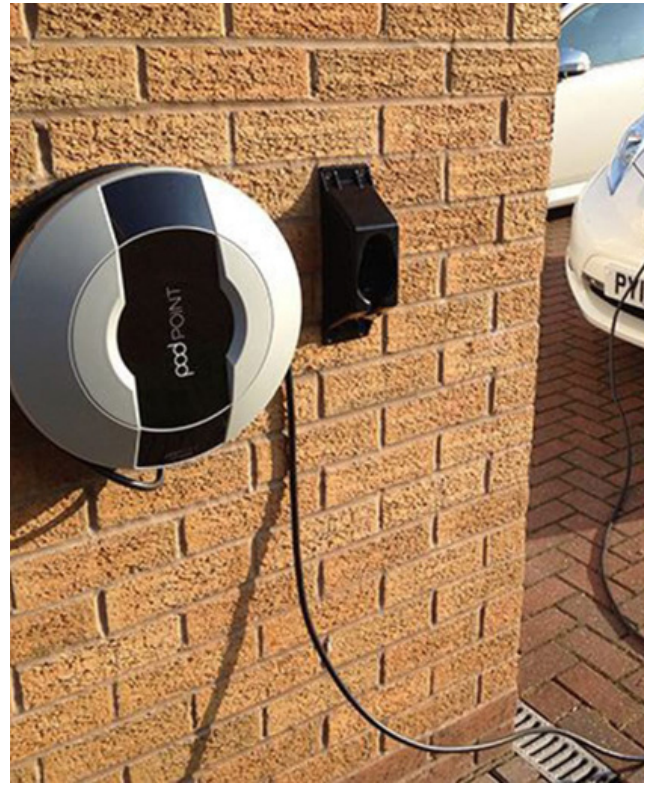
Figure 118: EV charging point
